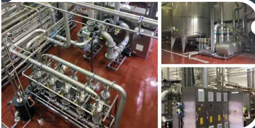
COCA COLA FACTORY WATER TREATMENT SYSTEM – 2022
